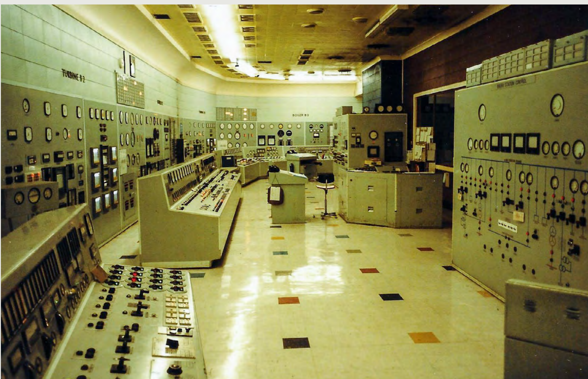
Staythorpe B Power Station control room
